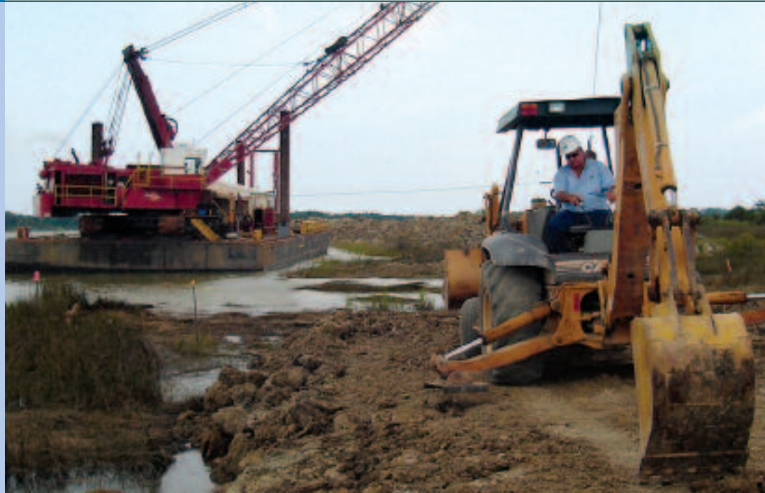
James Construction excavated more than 1 million cubic yards of soil from the Cameron LNG site.
